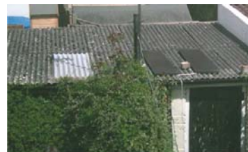
Solar panels on shed
